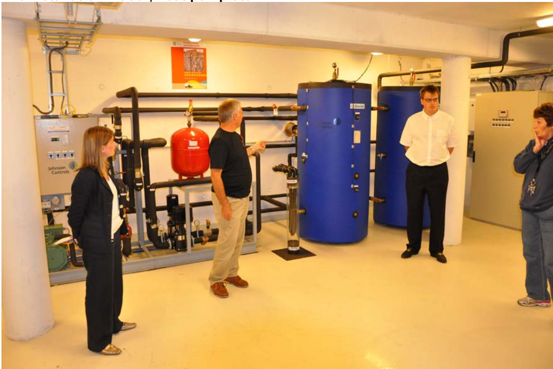
The installation indoor, heat pump etc.
